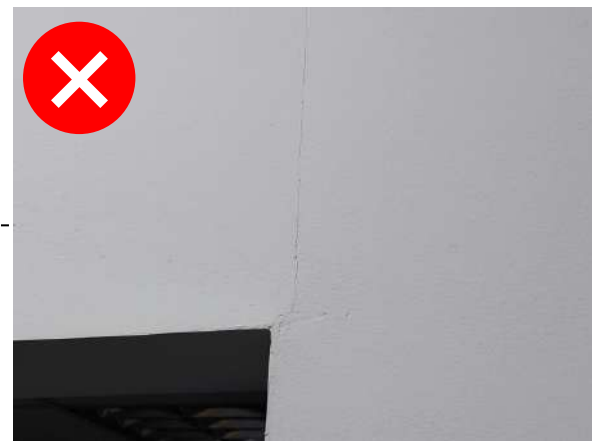
<Wall without JOINER> Random cracks
