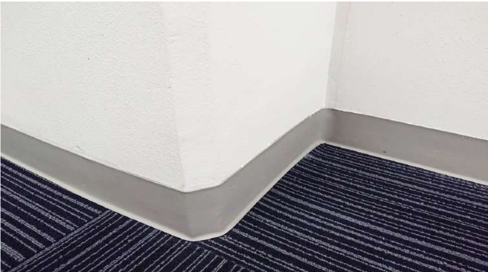
■ FACTORY OFFICE (DONG NAI/VIETNAM)
