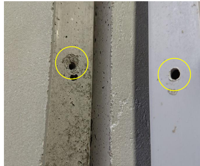
The appearance of the enlarged hole (Need repair)
